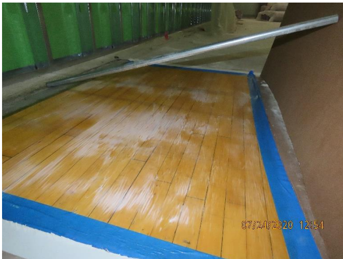
Armor Guard Protection of existing flooring (Potential exterior moisture/construction damage)
