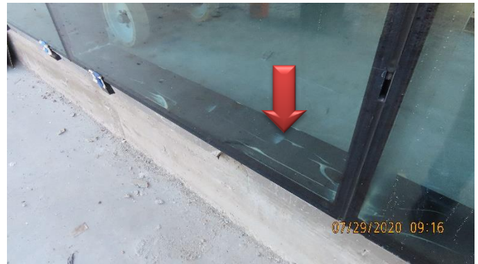
Armor Guard on and glass aluminum (interior) (Interior installation seen from the exterior)
