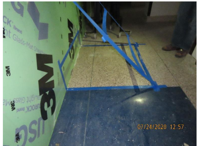
Armor Guard Protection of existing terrazzo (Potential exterior moisture/construction damage)
