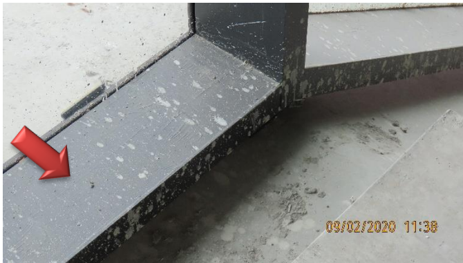
Concrete Splatter on aluminum & glass - protected with Armor Guard (concrete will damage aluminum & glass finishes)
